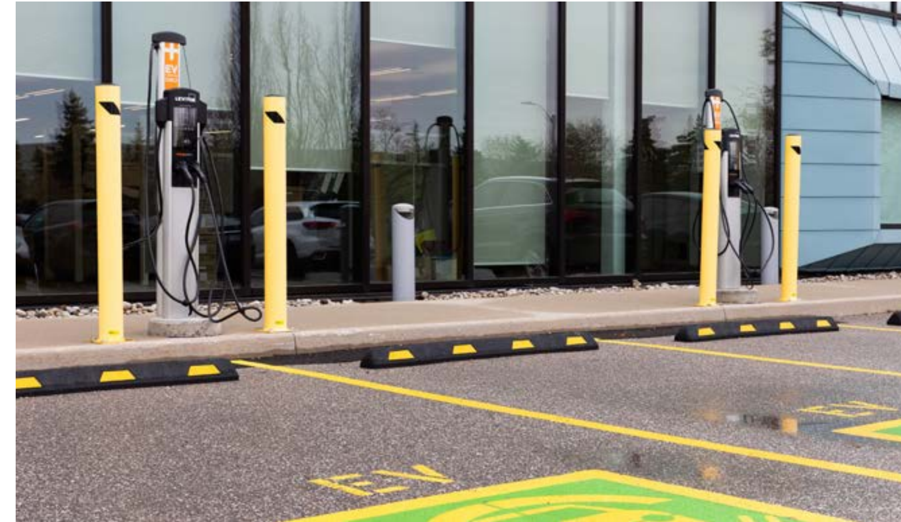
Charging stations for electric vehicles at our facility in Brampton, Ontario
